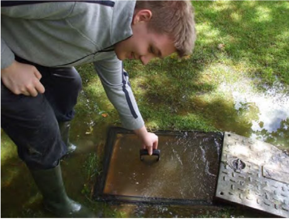
Figure 41 - Brooks Meadow - Adam inspecting flood water at drain cover
