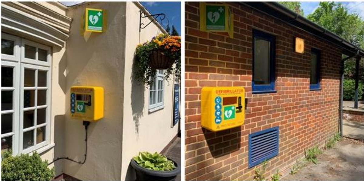
Image 3: Defibrillators installed by Winchfield Parish Council at the Barlow Mow (left) and Winchfield Village Hall (right) using funding received from S106 Planning Obligations.
