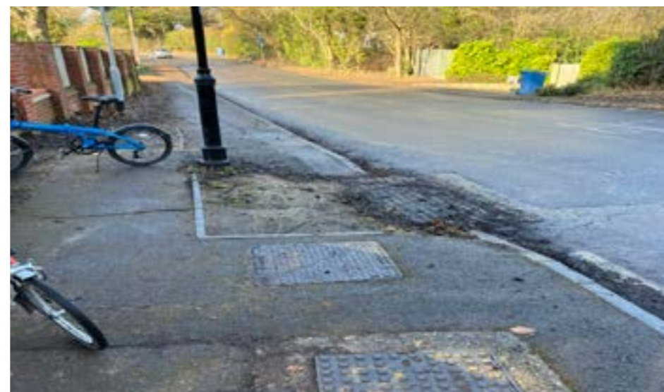
Poor crossing point at The Street / Crookham Road junction
