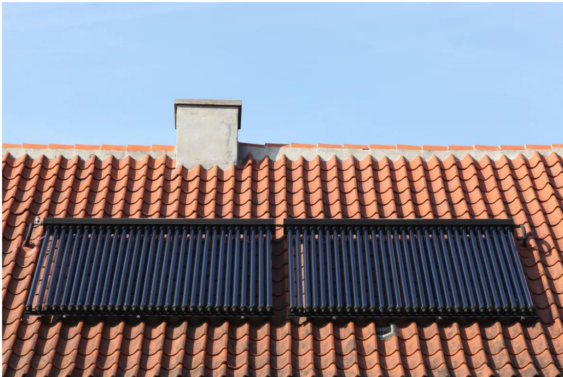
Image 5: Solar thermal panels on a roof (Image credit: Energy Saving Trust)
